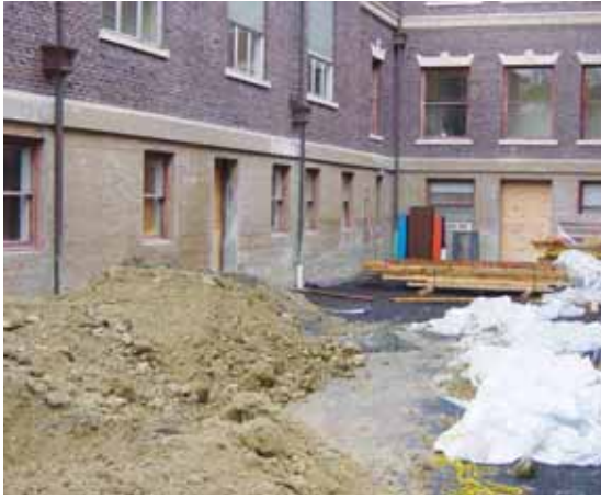
After Seattle Hebrew Academy sustained severe damage in a 2001 earthquake, the Orthodox Union challenged federal disaster relief regulations and lobbied for government funding on behalf of the school. As a result, the government awarded the school with over one million dollars in disaster assistance.
